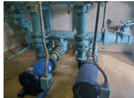
Figure 3-10 McFarland Booster Pumps
