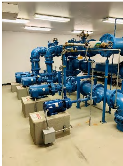
Figure 3-12 Coyote Booster Pumps
