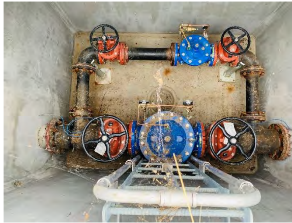
Figure 3-23 Monroe Street PRV Station
