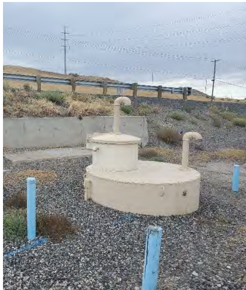
Figure 3-13 McNary Booster Station
