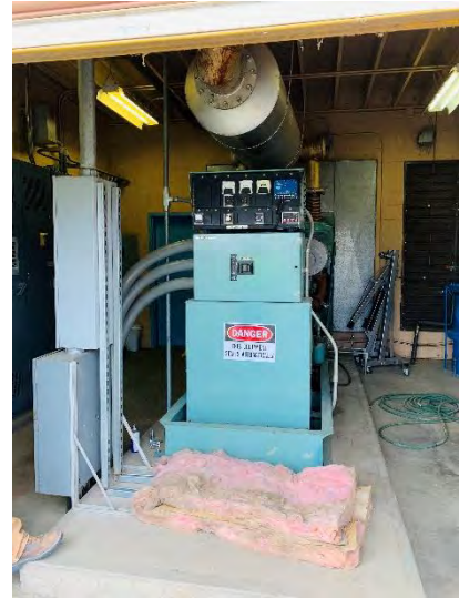
Figure 3-6 Golf Course Well Diesel Generator
