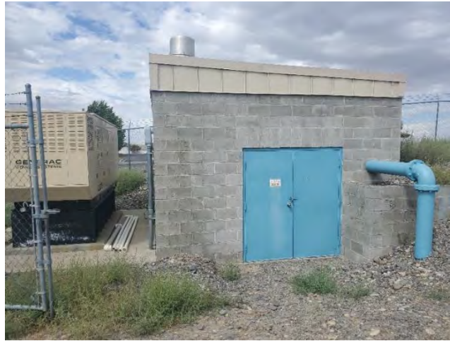
Figure 3-9 McFarland Booster Station
