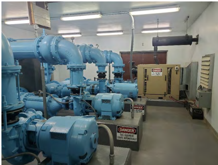
Figure 3-16 Golf Course Booster Pumps
