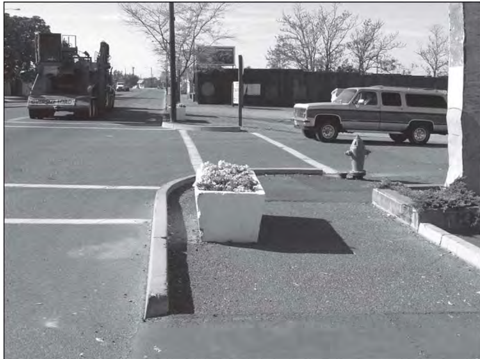
Missing or inadequate sidewalk segments, such as this at-grade corner behind an extruded curb, should be fixed.
