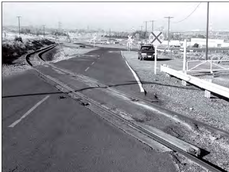
Angled tracks with a rough irregular flange opening can easily cause a cyclist to fall
